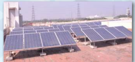
25 KW Solar Power Panel
