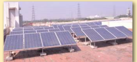
25 KW Solar Power Panel
